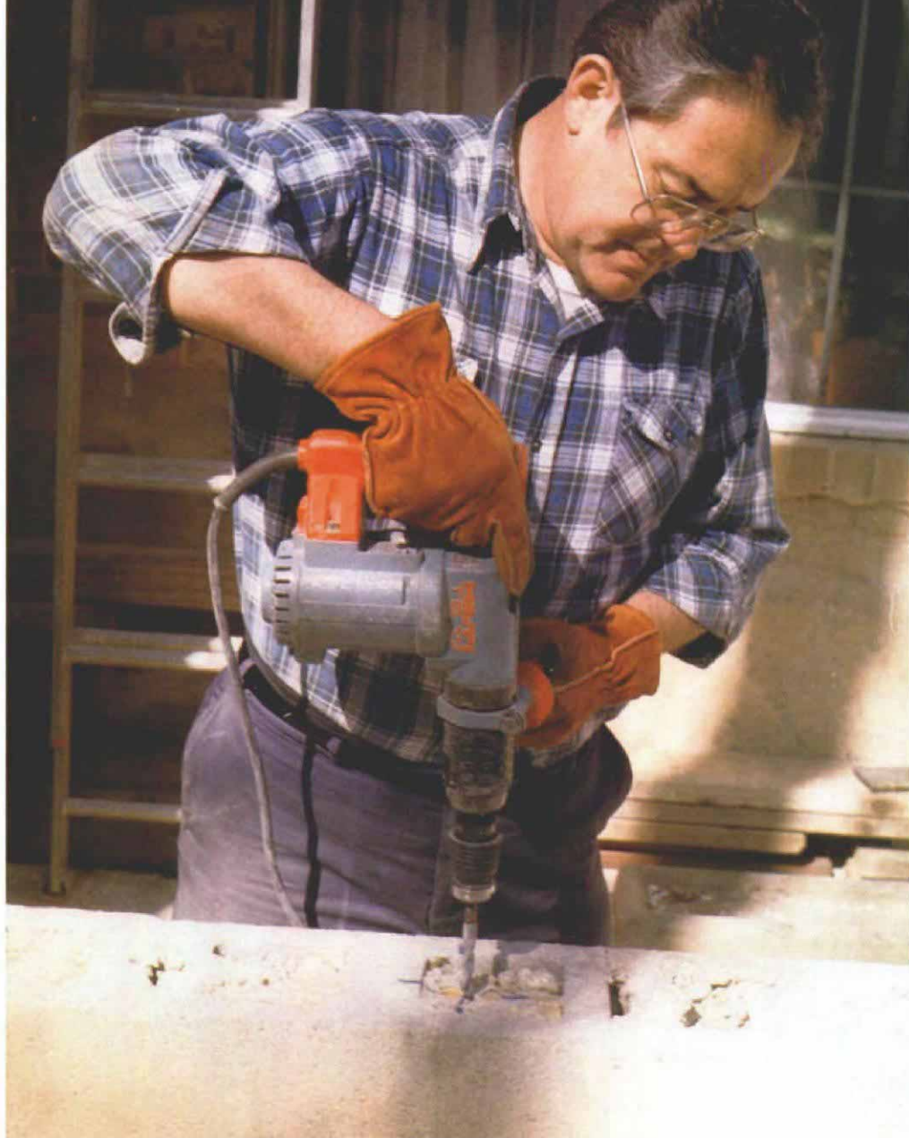
The deck rests partially on a concrete-block wall that had been built some years before, but with the later construction of the deck in mind. The cores of the block had been reinforced and poured solid, so holes had to be hammer-drilled into the concrete for the anchor bolts (as shown in this photo), which were later grouted in place.
