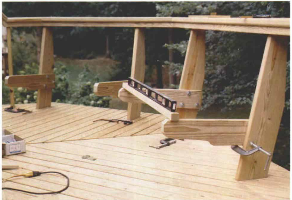
Installing benches single-handed can be tough, but the liberal use of clamps can speed the job. The bench backs and seats were angled slightly to make them more comfortable.
