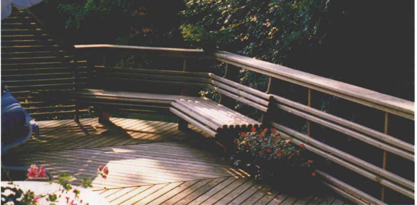
The completed deck includes herringbone decking and a privacy screen at one end. Note the rounded front portion of the benches, a detail designed to increase comfort. Edges on the benches and on the railing were sanded smooth.
